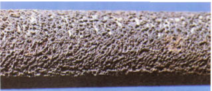
Figure 17.13 Erosion on mild steel turbine drain line. Surface is festooned with small, conical projections pointing toward the direction of impingement.
