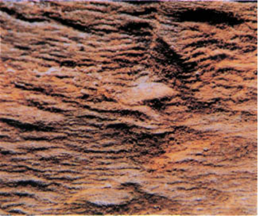
Figure 17.4 Finely spaced, wavelike, parallel undulations on eroded fire-side external surface of superheater tube. The striations resemble waves viewed from the air and are aligned perpendicularly to the direction of steam impingement. (Compare with Fig. 17.3.)
