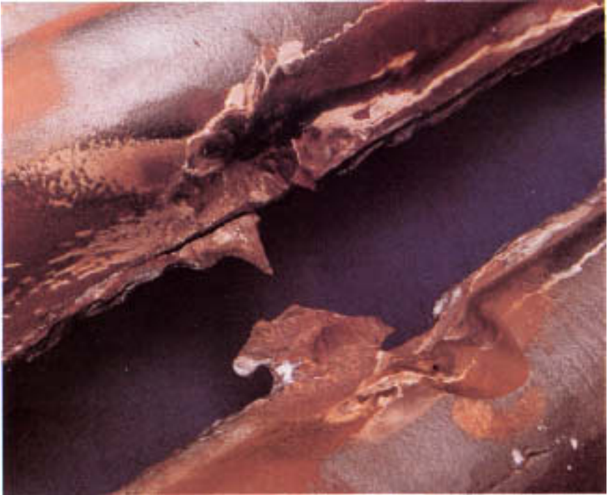
Figure 17.20 Steam cutting of utility convection tubes. The original failure occurred at a welded support bracket and was due to corrosion fatigue. The adjacent tube was breached by escaping steam from the original failure.
