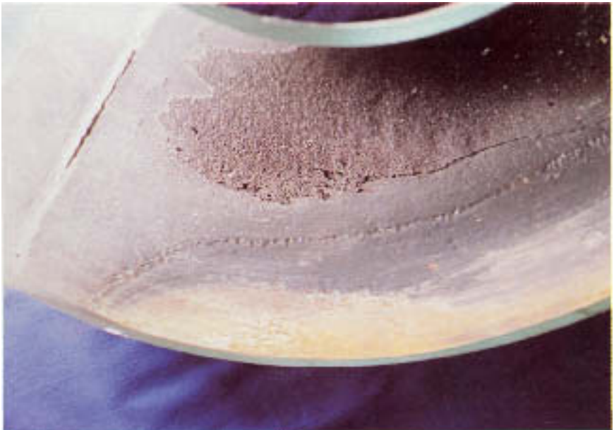
Figure 17.17 Localized metal loss in a bend of a condensate return header.
