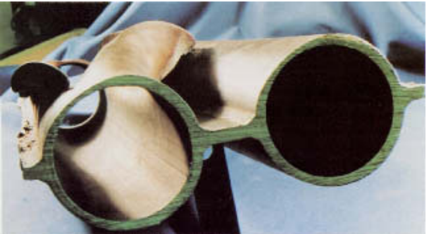
Figure 17.16 Ruptured division-wall tube from fluidized-bed boiler. Attack was caused by sand abrasion in the bed.
