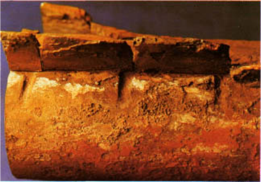
Figure 17.8 Deep grooves cut into the hot side of a waterwall tube. Grooving was caused by channeling of furnace gases containing entrained fly ash.
