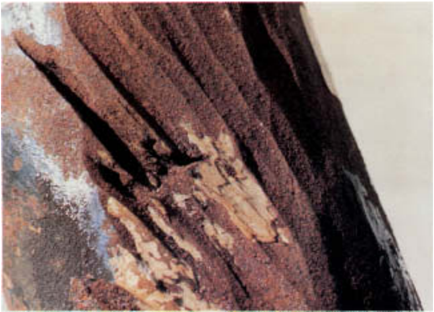
Figure 17.6 Grooving on pendant U-bend superheater leg caused by steam leaking through a corrosion-fatigue crack at the U-bend. Grooves were rusted after removal from boiler.
