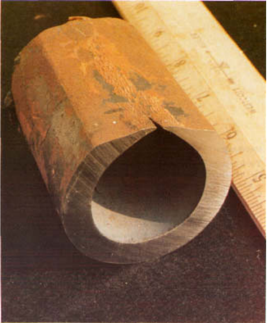
Figure 17.1 Superheater section thinned by soot-blower erosion. Note the flattened surface. The tube bulged and ruptured on the thinned side. Also, note how the eroded surface color is not dissimilar to unattacked regions, indicating intermittent attack.
