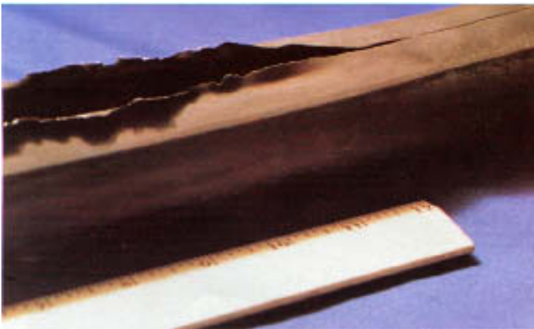
Figure 17.2 Tube rupture caused by a misdirected soot blower. Rupture edges are thin and ragged because of tearing of the wasted steel in the eroded zone. The tube surface is light gray and shiny as a result of erosion of the normally present fire-side oxides and deposits.
