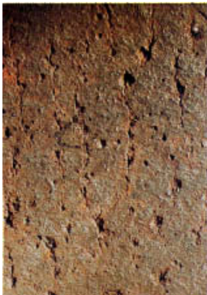
Figure 15.5 Transverse cracks and associated oxygen pits.
