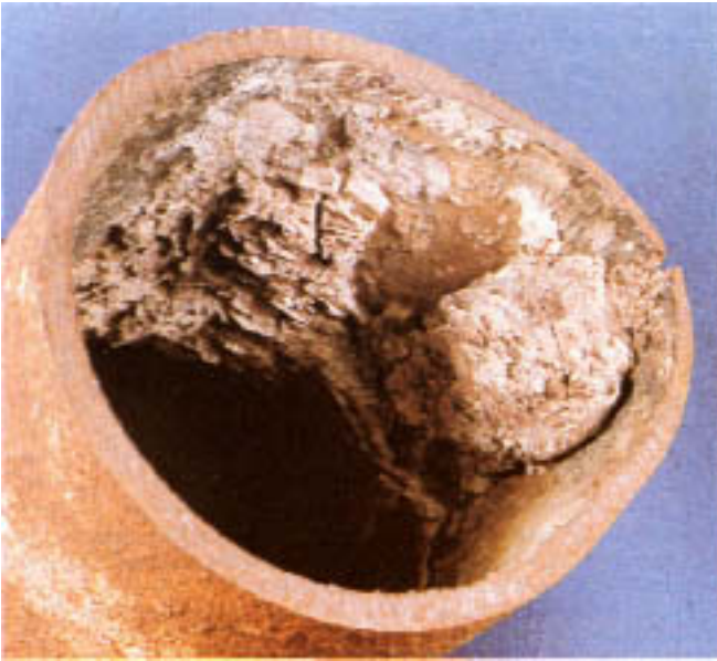
Figure 1.11 Sodium hydroxide-rich deposit on fire side of wall tube from 600-psi boiler. Note the bulge due to long-term overheating.
