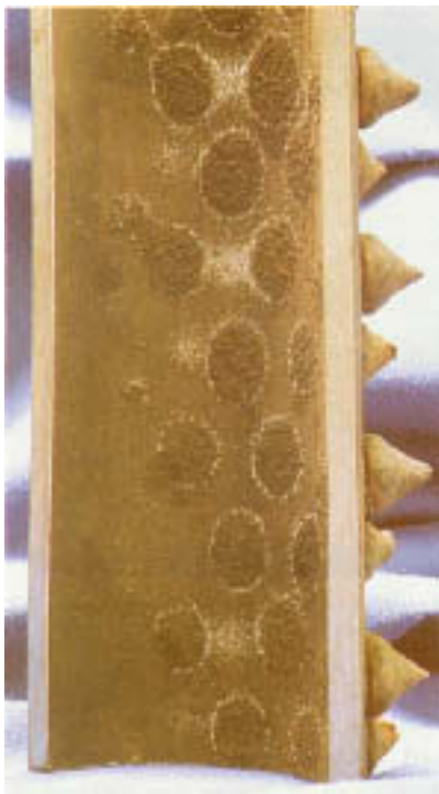
Figure 1.14 Spots of particulate iron oxide deposit mirroring stud locations on a wall tube of a recovery boiler. The studs, if exposed, concentrate heat, causing higher rates of steam generation and deposition. Note the white deposits of sodium hydroxide encircling each powdery magnetite spot.
