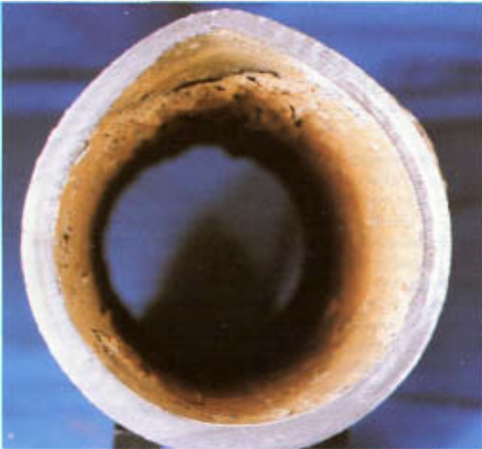
Figure 1.24 Cross section of bulged target-wall tube. Deposits are heavy on both hot and cold sides. Most deposits are phosphates, silicates, and carbonates.
