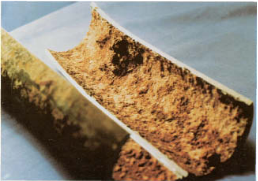
Figure 1.4 Thick layer of friable iron oxide in an economizer tube. Most iron was carried into the economizer from the preboiler system.
