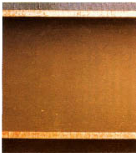
Figure 1.13 Smooth, tenacious, black, magnetite layer on a well-protected boiler tube.
