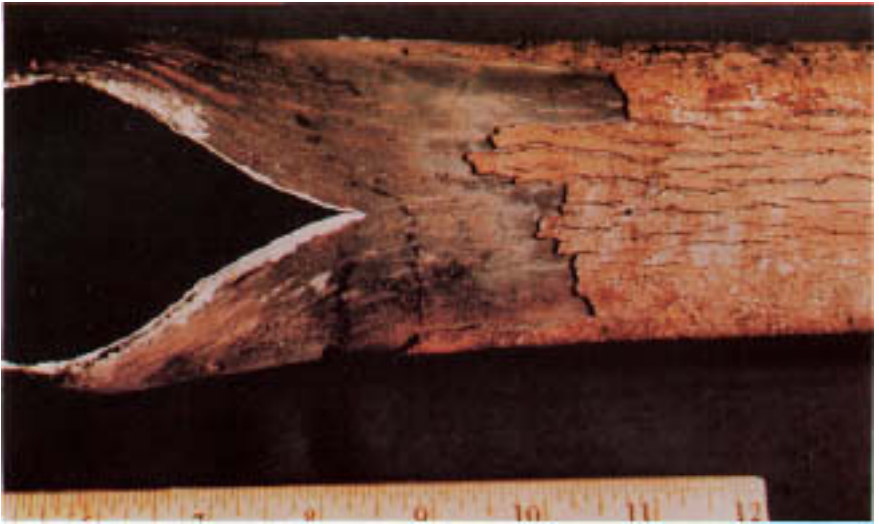
Figure 2.5 Thermally deteriorated metal on failed wall tube of a utility boiler. Note the spalled and cracked oxide resembling tree bark caused by expansion of tube during bulging and thermally induced stresses.
