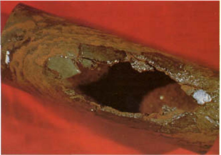
Figure 2.6 Through-wall oxidation of a tube from a low-pressure boiler. Brittle black magnetite patches still adhere to the rupture mouth. Elsewhere the oxide has spalled. Such through-wall oxidation is most common in low-pressure boilers, where internal pressures are not sufficient to cause premature failure.
