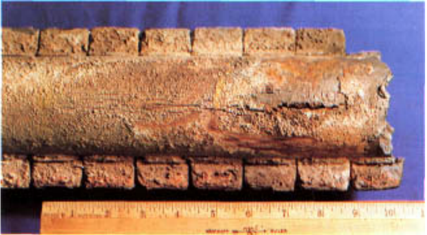
Figure 2.12 Longitudinal fissures along hot side. Note the through-fissure at the bulge apex.
