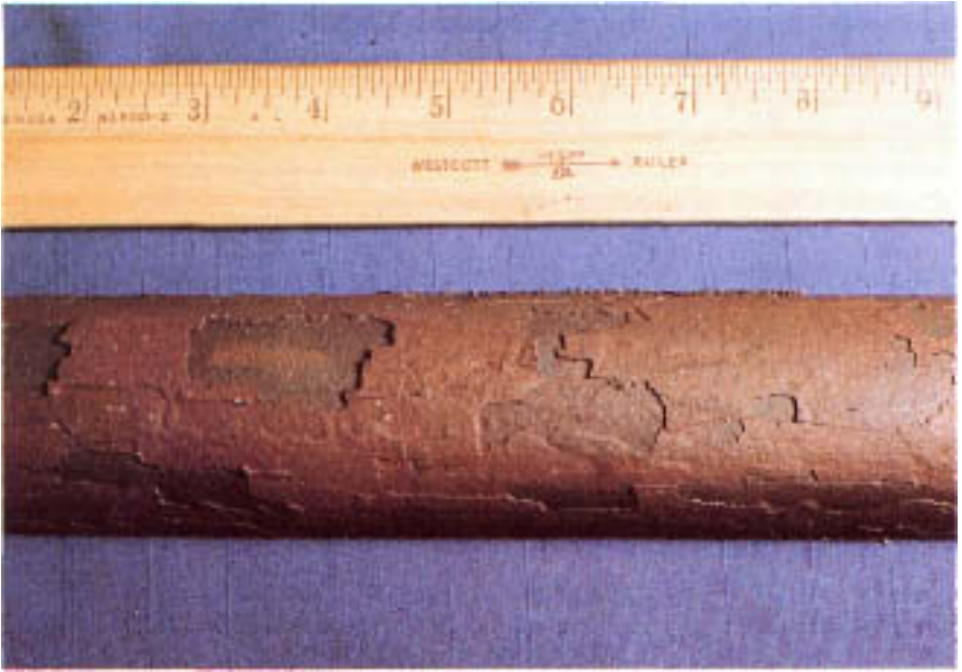
Figure 2.11 Severe thermal oxidation and spalling of magnetite on external surface. The laminated nature of the scale indicates multiple episodes of spalling and oxide reformation.
