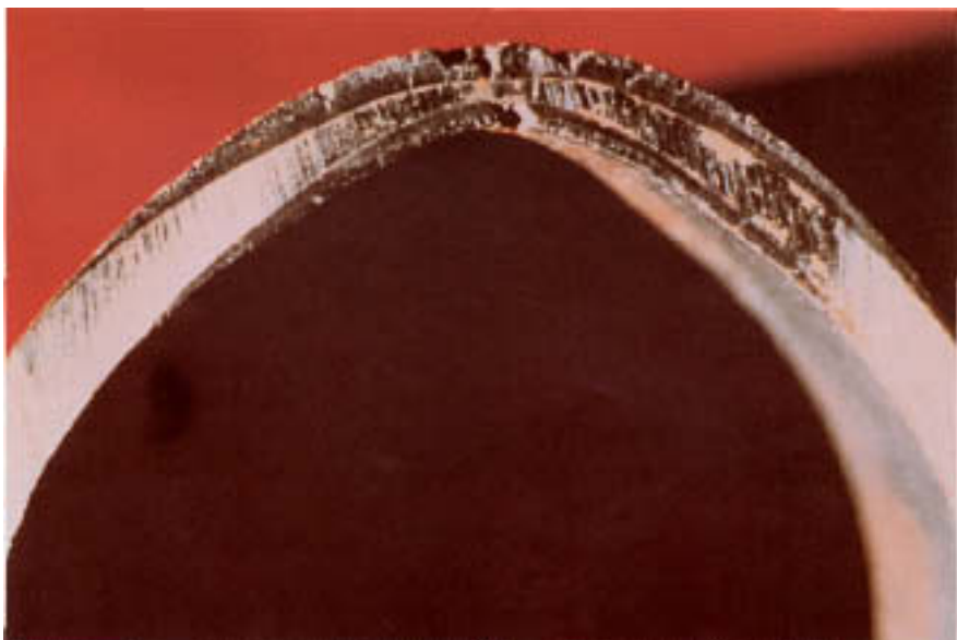
Figure 2.3 Thick, thermally formed oxide on internal and external surfaces of a bulged wall tube. Thinning of intact metal at bulge is due to both plastic deformation and thermal oxidation.
