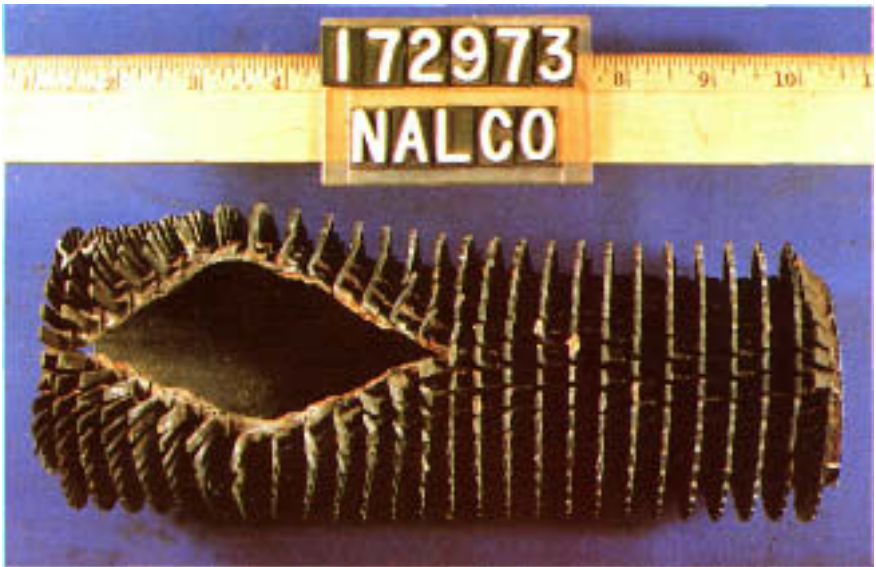
Figure 3.7 Large, wide-open rupture in a superheater tube of a waste-heat boiler. The tube experienced long-term overheating followed by a brief episode of short-term overheating when nearby tubes ruptured.
