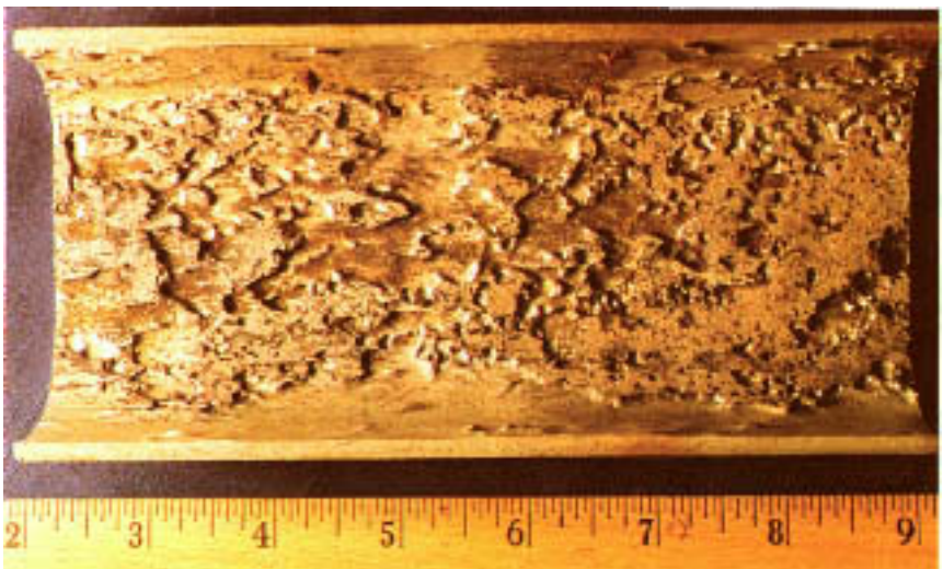
Figure 5.2 Chelant corrosion altered by the presence of excessive oxygen.
