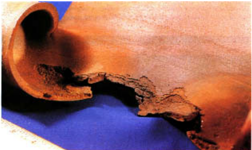
Figure 6.4 Metal loss at the origin of rupture.
