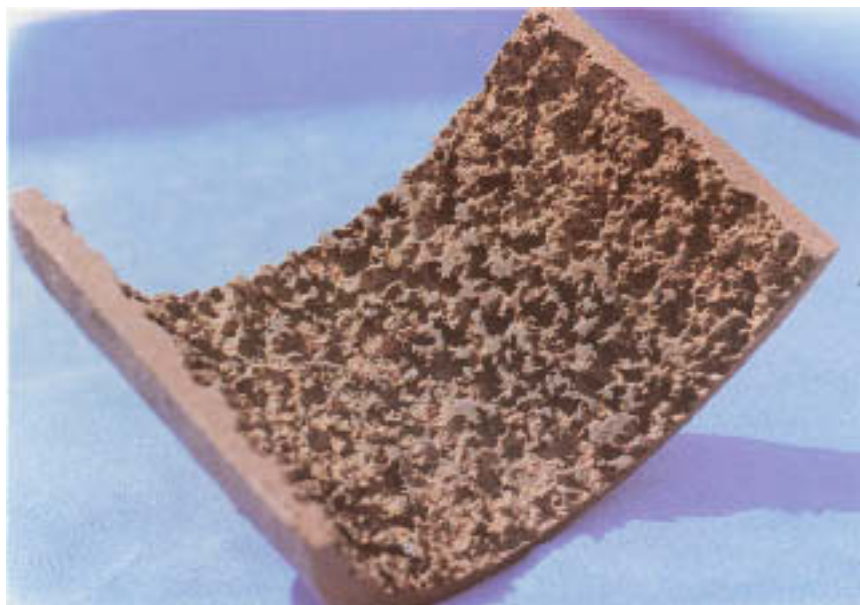
Figure 7.4 Jaggedness associated with severe acid corrosion. (Courtesy of Electric Power Research Institute.)
