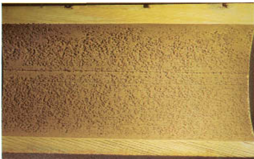
Figure 7.1 Acid corrosion on the internal surface of a wall tube. (Courtesy of Electric Power Research Institute.)
