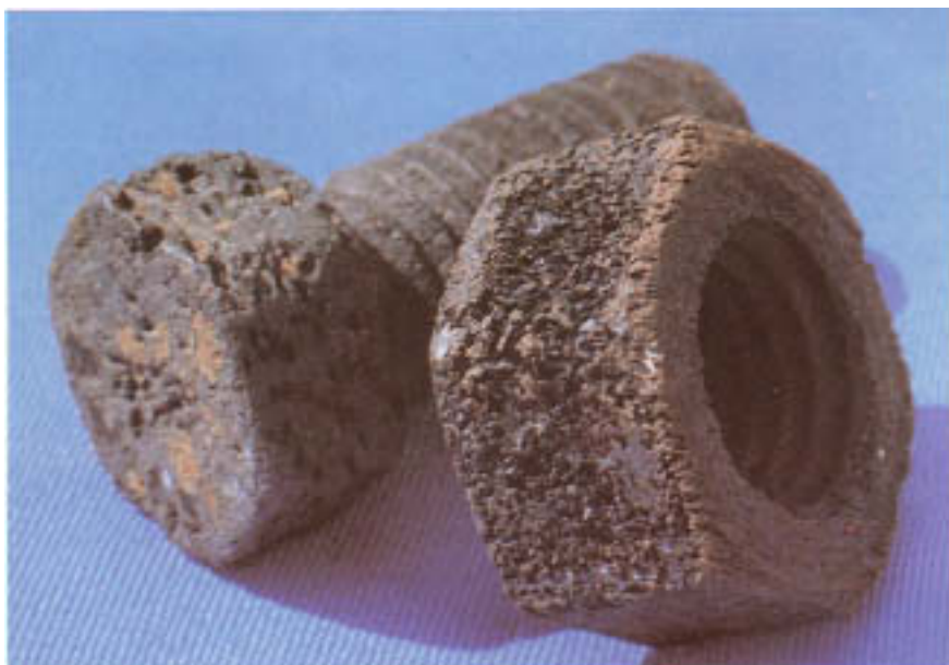
Figure 7.3 Acid corrosion of attachment hardware.
