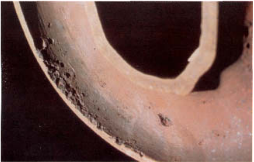
Figure 8.3 Oxygen pits along bottom of superheater pendant. (Courtesy of National Association of Corrosion Engineers.)
