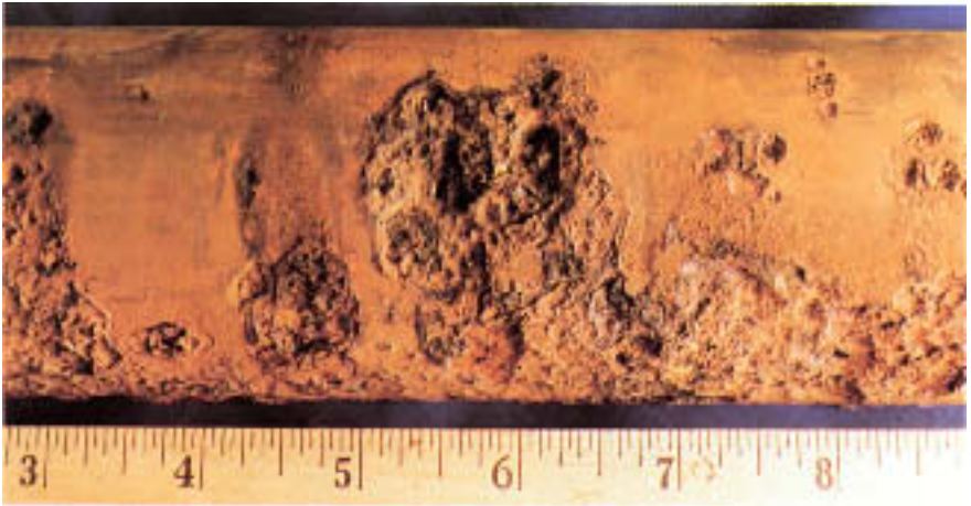
Figure 8.8 Oxygen pitting on the external surface of fire tube.
