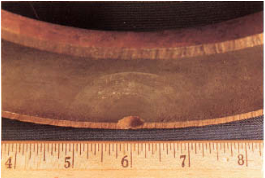
Figure 8.4 Elliptical water rings surrounding oxygen pit in a U-bend. (Courtesy of Electric Power Research Institute.)
