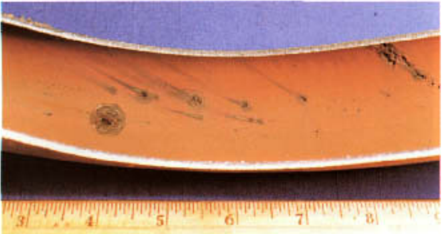
Figure 8.5 Oxygen pits on internal surface.
