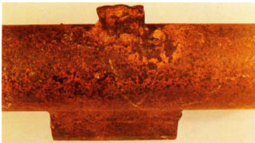
Figure 9.6 High-temperature corrosion at the base of an attachment (top of photograph) on a stainless steel reheater tube. (Courtesy of Electric Power Research Institute.)
