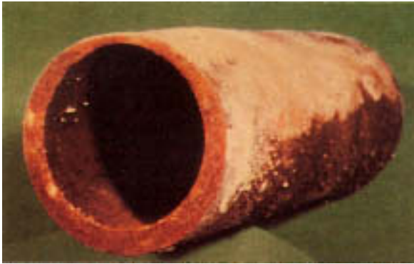
Figure 9.4 Wall thinning from oil-ash corrosion. Corrosion rates of 30 mil/y (0.76 mm/y) have been observed. (Courtesy of Electric Power Research Institute.)
