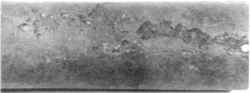
Figure 9.5 Oil-ash corrosion on stainless steel reheat tube. (Courtesy of John Wiley and Sons, Metallurgical Failures in Fossil Fired Boilers , by David N. French, New York, 1983.)
