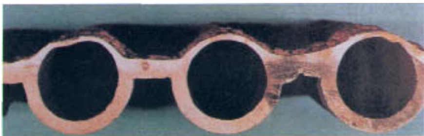
Figure 11.2 Severe fire-side metal loss on waterwall tubes. (Courtesy of Electric Power Research Institute.)
