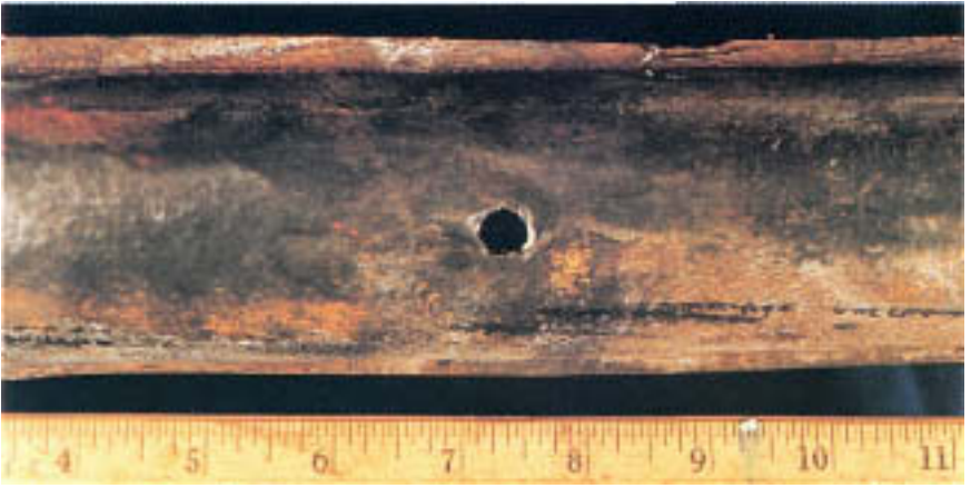
Figure 11.5 Perforation in a region of severe metal loss.
