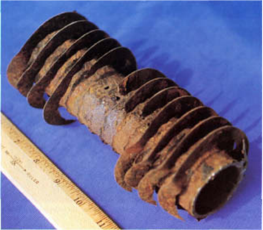
Figure 12.4 Corrosion and perforations of finned economizer tube resulting from exposure to condensed sulfuric acid. Note detachment of fins from tube wall.
