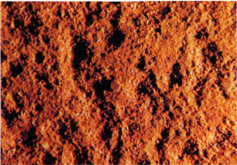
Figure 12.3 Pockmarked contour of economizer tube exposed to condensed sulfuric acid. (Magnification: 7.5X.)
