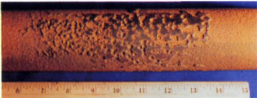
Figure 13.6 Corrosion resulting from inadequate water washing of external surfaces.
