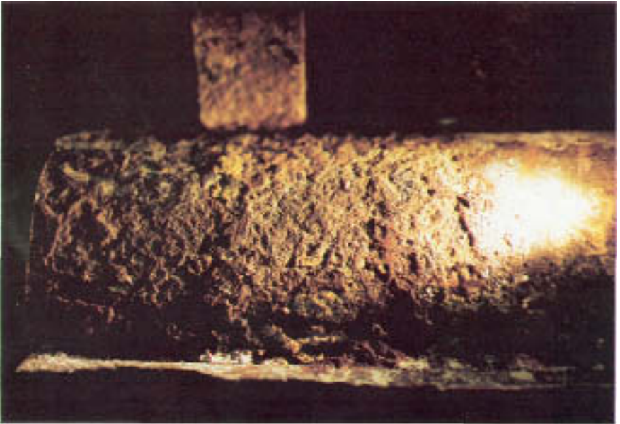
Figure 13.5 Idle-time corrosion occurring beneath refractory.
