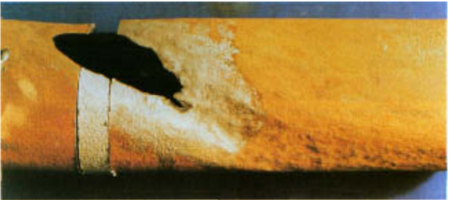
Figure 13.7 Grooving and perforation of a slanted tube resulting from corrosive water dripping from above.
