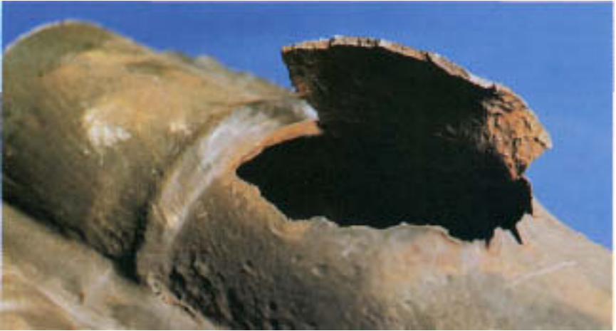
Figure 14.4 Rupture resulting from hydrogen damage. Note proximity of failure to circumferential weld. (Courtesy of Electric Power Research Institute.)
