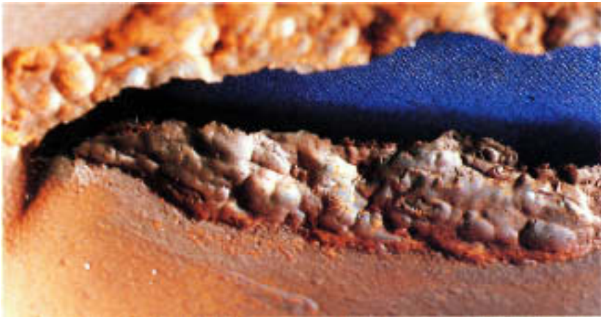
Figure 14.6 Smooth, wavelike contours of internal surface resulting from caustic gouging.
