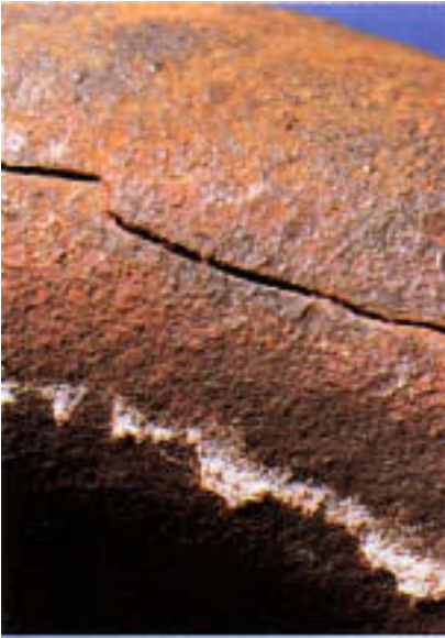
Figure 16.4 Longitudinal crack along the side of a 90° bend in an economizer tube. A similar crack is located along the opposite side.
