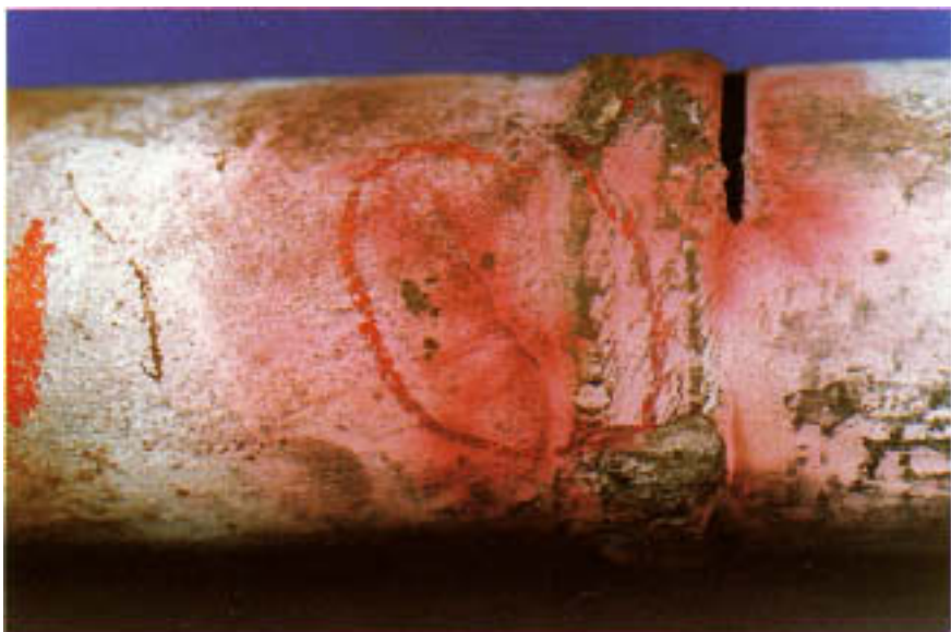
Figure 16.5 Appearance of stress-corrosion crack on the external surface. Crack is located within the red circle.
