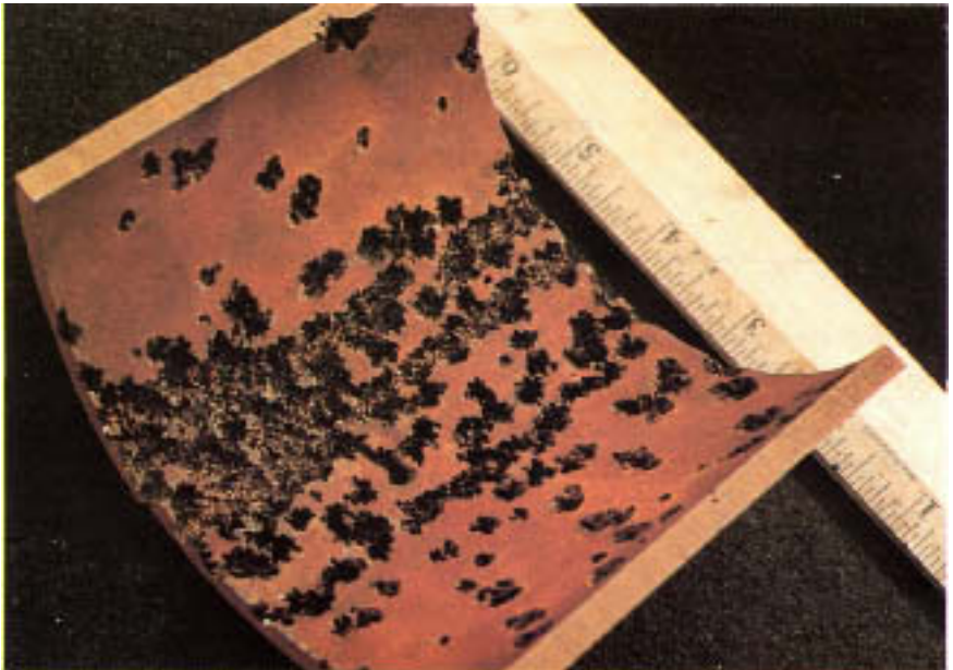
Figure 18.6 Heavily pitted condensate line. Attack resembles oxygen pitting, but was caused (at least in part) by cavitation.
