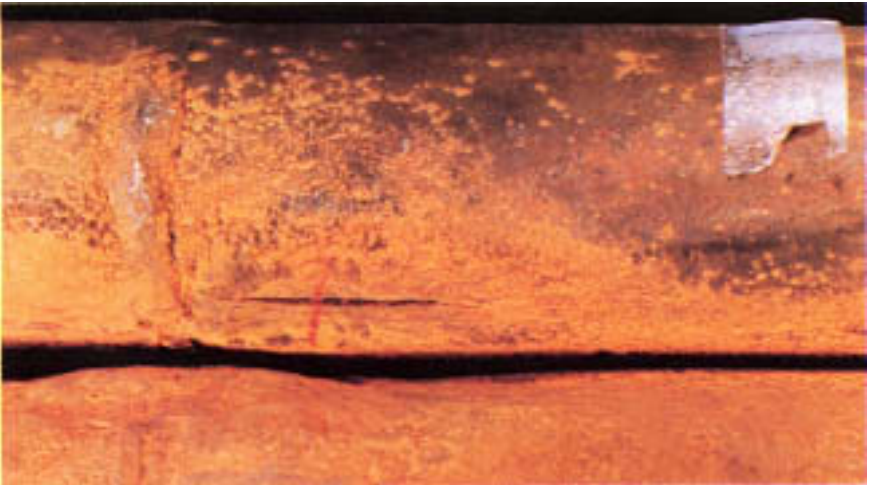
Figure 19.2 Seam defect (top tube). External metal loss on the bottom tube is the result of erosion from mixed steam and water escaping through the rupture.
