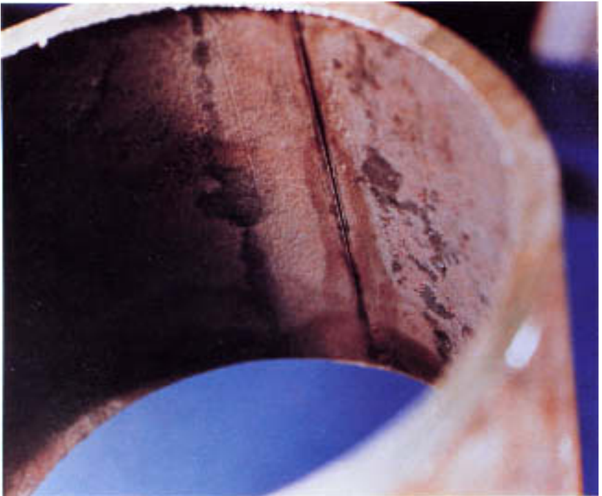
Figure 19.8 Seam defect in steam line.
