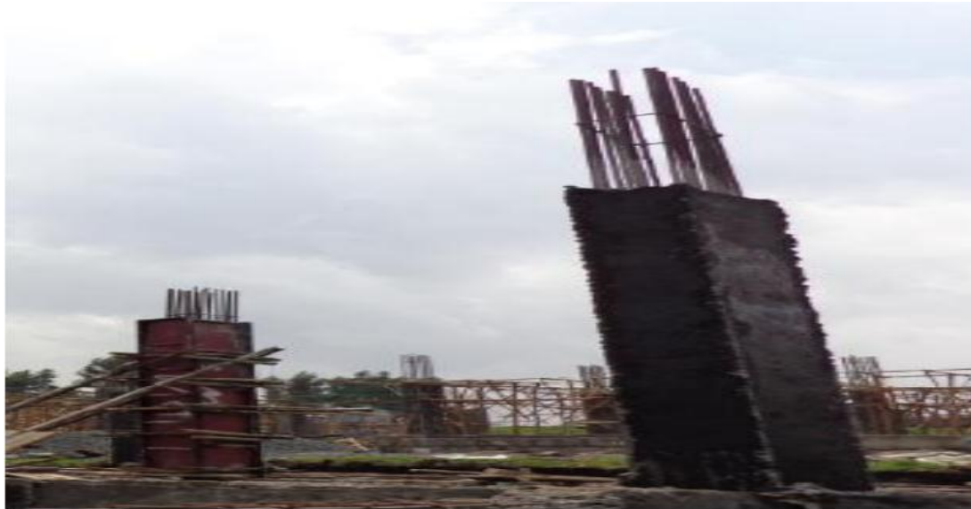
Figure 4.9: Column after stripping of steel formwork some roughness and discoloration on concrete surface at bole site.
