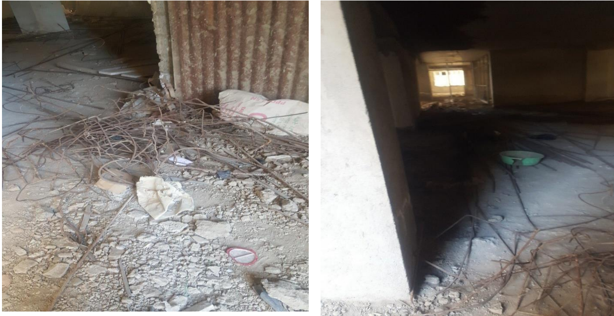
Figure 4.3. improper handling of reinforcement bar
