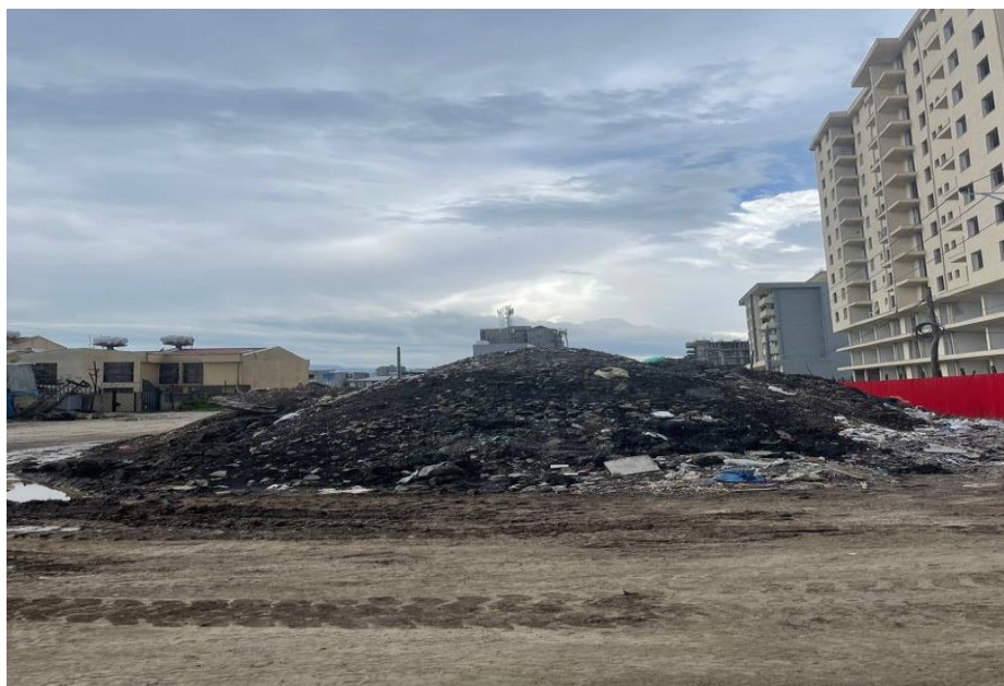
Figure 4.2. improper dumping excavated soil
