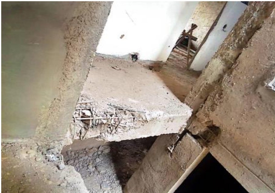
Incomplete Electrical Duct
