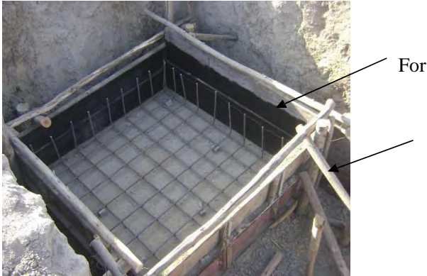
Figure 2. 7 Footing pad formwork construction system in Addis Ababa (Gerji Federal Housing Project)
