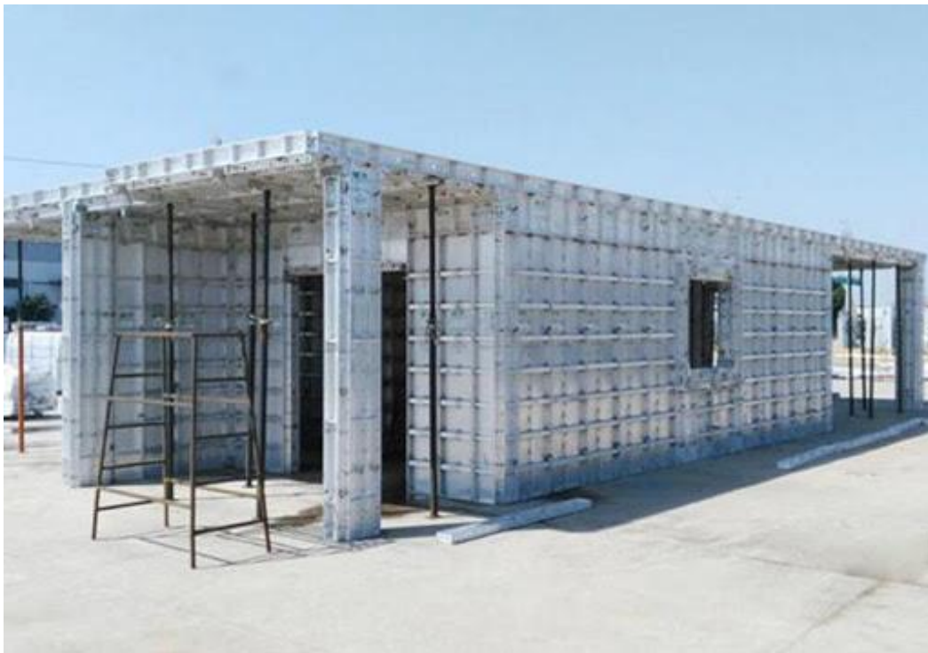
Figure 2. 2 Installation system of aluminum Formwork System (Kumkang Kind Formwork production Company Manual)
