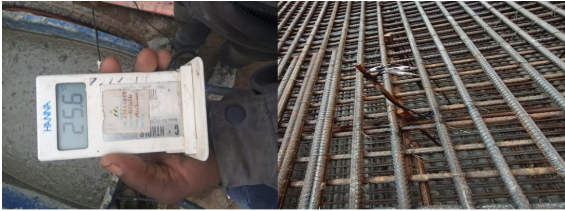
Fig 4. 12. The way of thermal heat of hydration control on site source: prepared by researcher.
