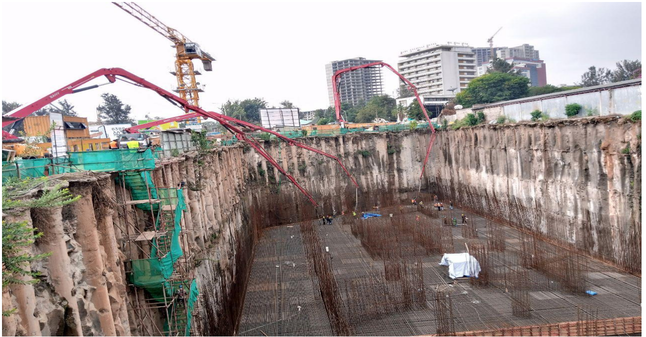
Fig 3. 3. Oromia Insurance headquarters project. source: prepared by researcher
