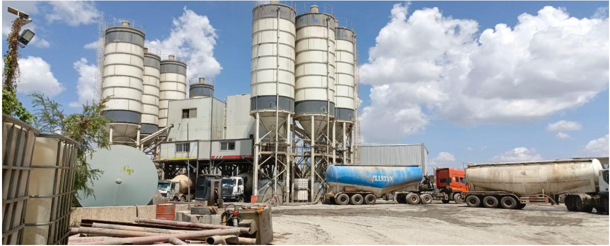
FIG 4.6 cement storage source: prepared by researcher
