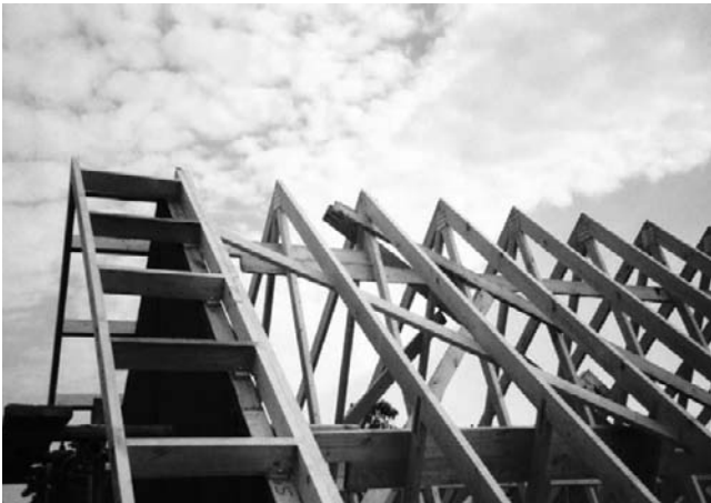
Figure 3.26 A trussed roof with diagonal wind bracing and showing a gable ladder (left of picture)
