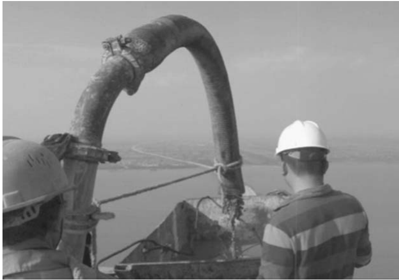
Figure 3-20 Pumping of fiber-reinforced concrete to a height of 306 m at Su-Tong Bridge, Suzhou, China (photo provided by Jinyang Jiang)
