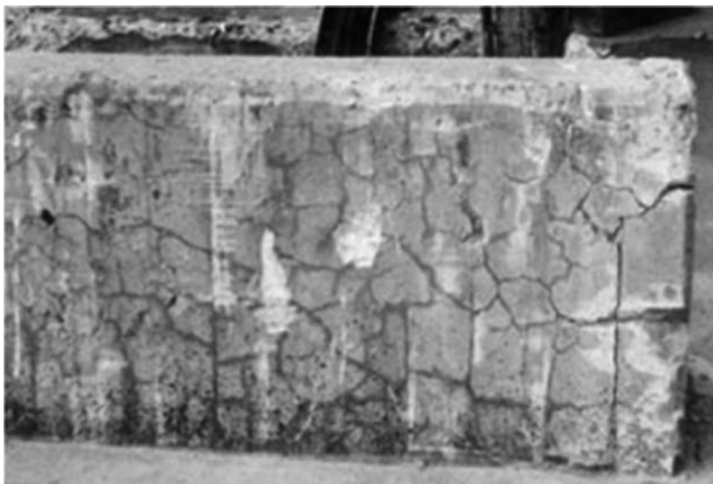
Figure 5-72 Cracks caused by AAR
