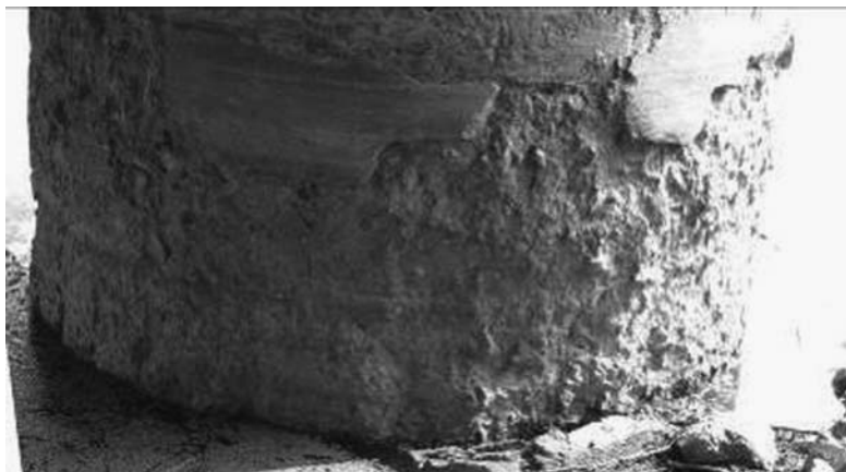
Figure 5-74 Scaling deterioration caused by freezing-thawing
